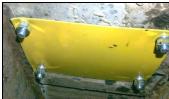
Figure 8: Bearing plate for tank bracket bolts.
